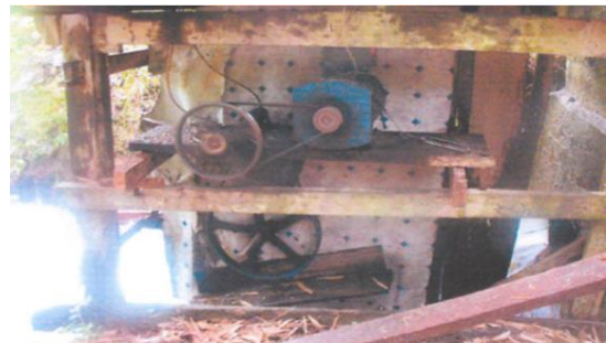
Figure 8. Construction of MHPP in Dusun III Kawerewere Source: Balitbang ESDM, Moving Toward Renewable Energy , (Jakarta: Balitbang ESDM, 2014), p. 27.
