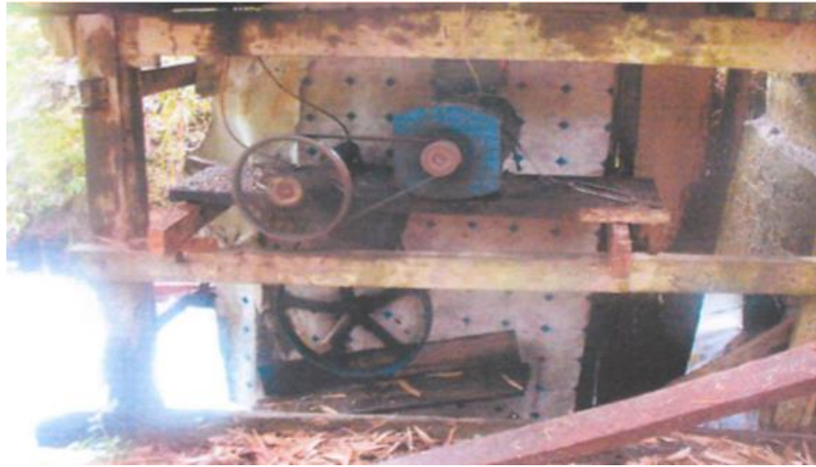
Figure 12. Construction of MHPP in III Kawerewere Village Source: R & D ESDM, Moving with Renewable Energy , (Jakarta: R & D ESDM, 2014), p. 27.
