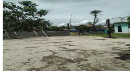
Coordinate: 5°43'41.6''S. 105° 35'51.2''E Fields condition: Settlement
